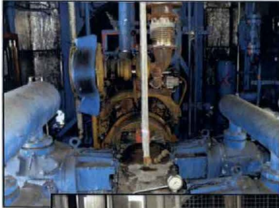
Original CNG Engine
