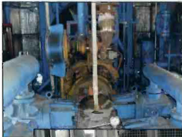
Original CNG Engine
