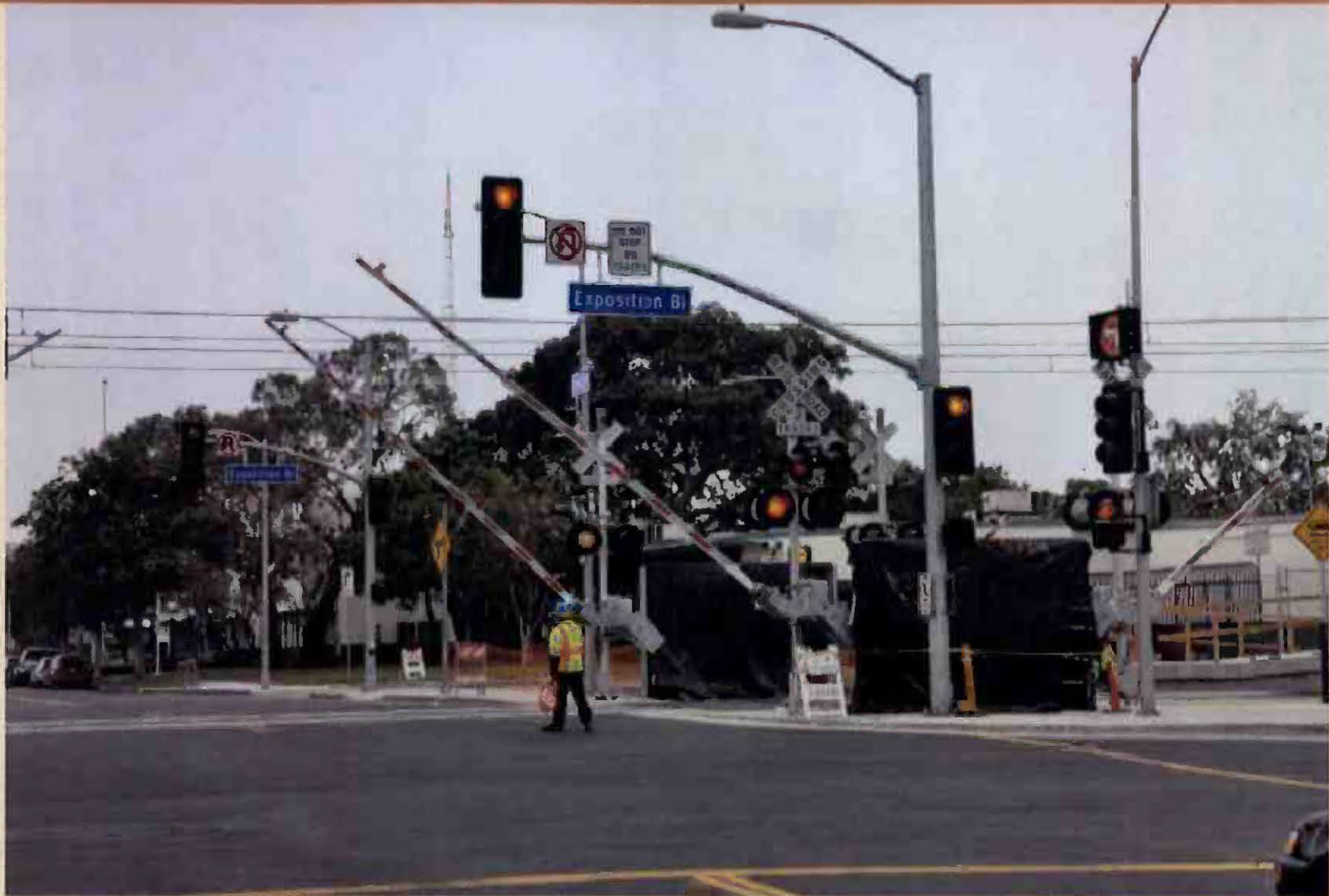
Testing of Gated Crossing at Farmdale Ave
