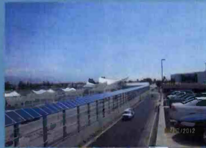
Screen wall and solar panels
