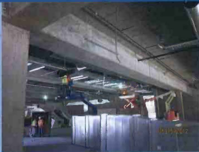
HVAC Ducting in Concourse
