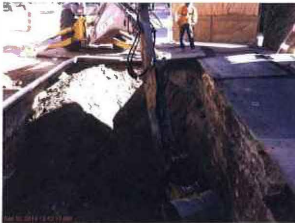
Advanced Utility Relocation - Removing sewer lateral and clay pipe on Flower St.
