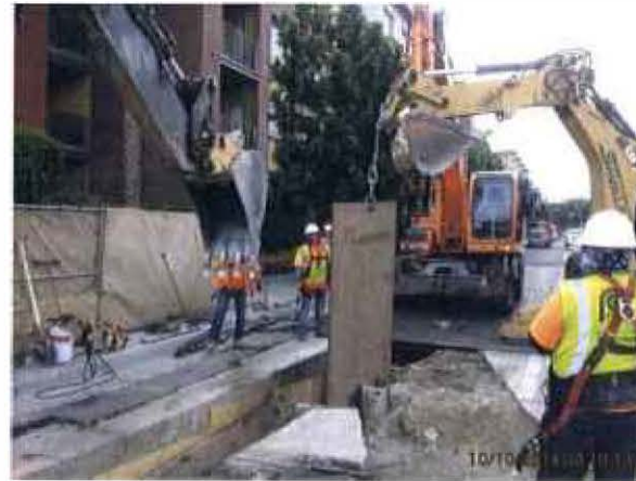
Advanced Utility Relocation – Setting a steel plate in trench on Alameda St.
