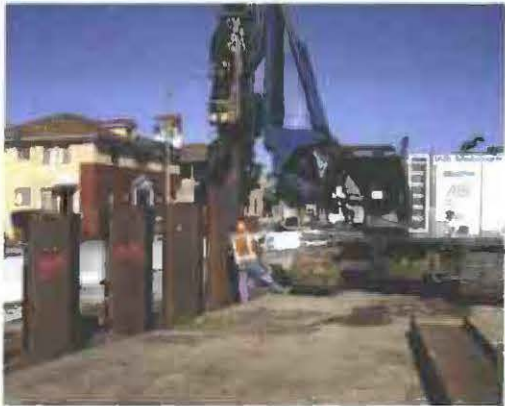
B2 – Vibrating piles at UG3 looking north (near Crenshaw and 58 th Place)
