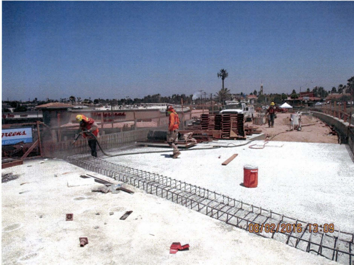
LA BREA BRIDGE – Preparation of the bridge deck for the upcoming parapet and emergency walkway work.
