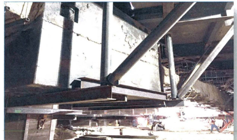
Hanging Utilities under Wye
