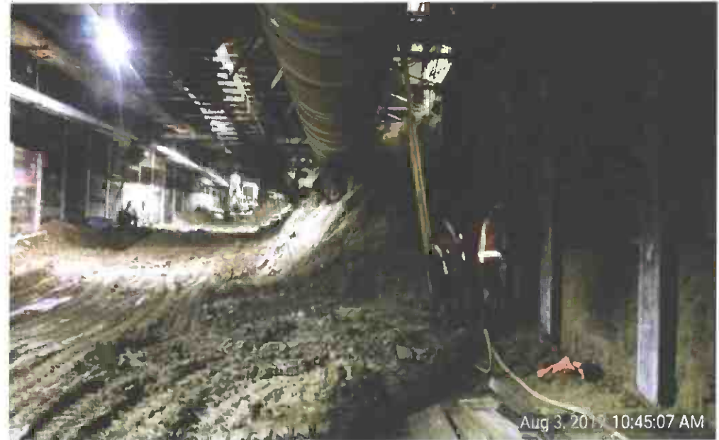
Excavation and lagging on east wall to elevation 268' just north of Access Shaft
