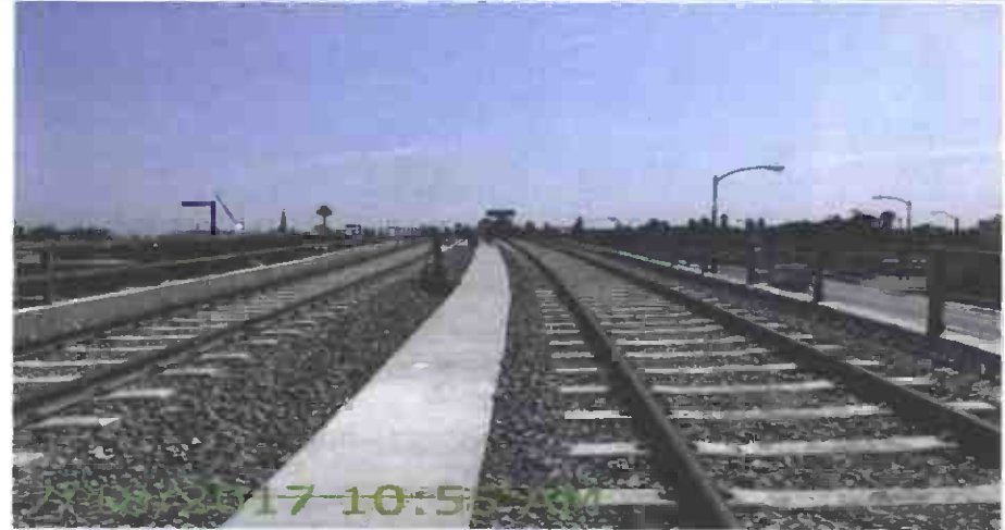
MSE 192 – Wall near La Brea bridge complete, ballasted track work in-place (surface and line and de-stressing complete)
