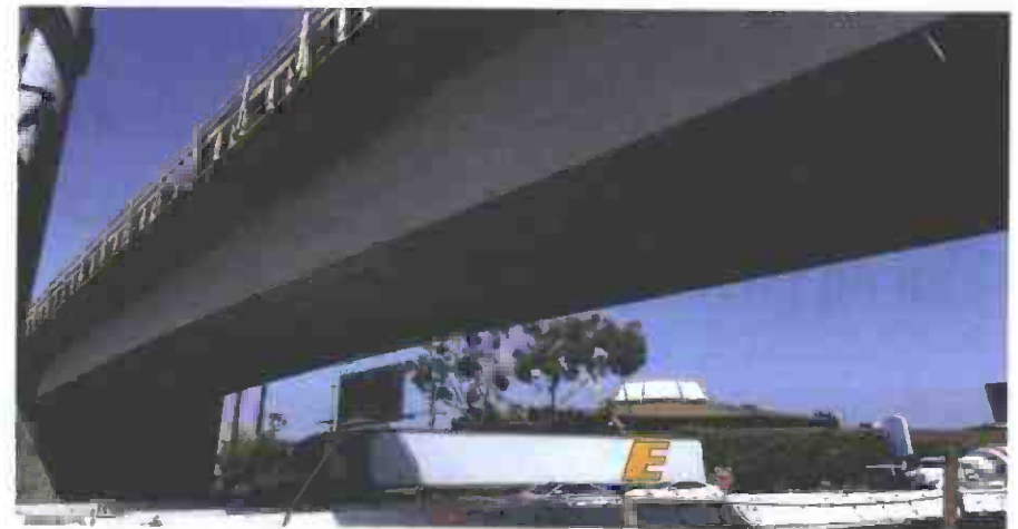
I-405 Bridge – Crews continued stripping formwork and finish work along the exterior girder stems.
