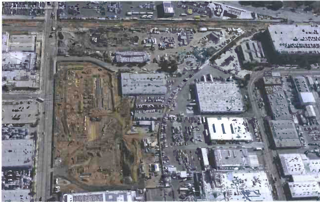
Aerial view of construction site on the left and the alignment work at the top.
