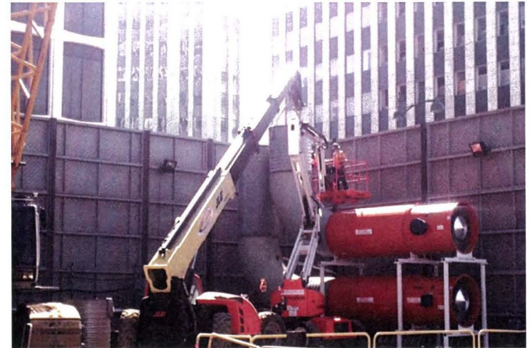
Wilshire/Western Site Ventilation System
