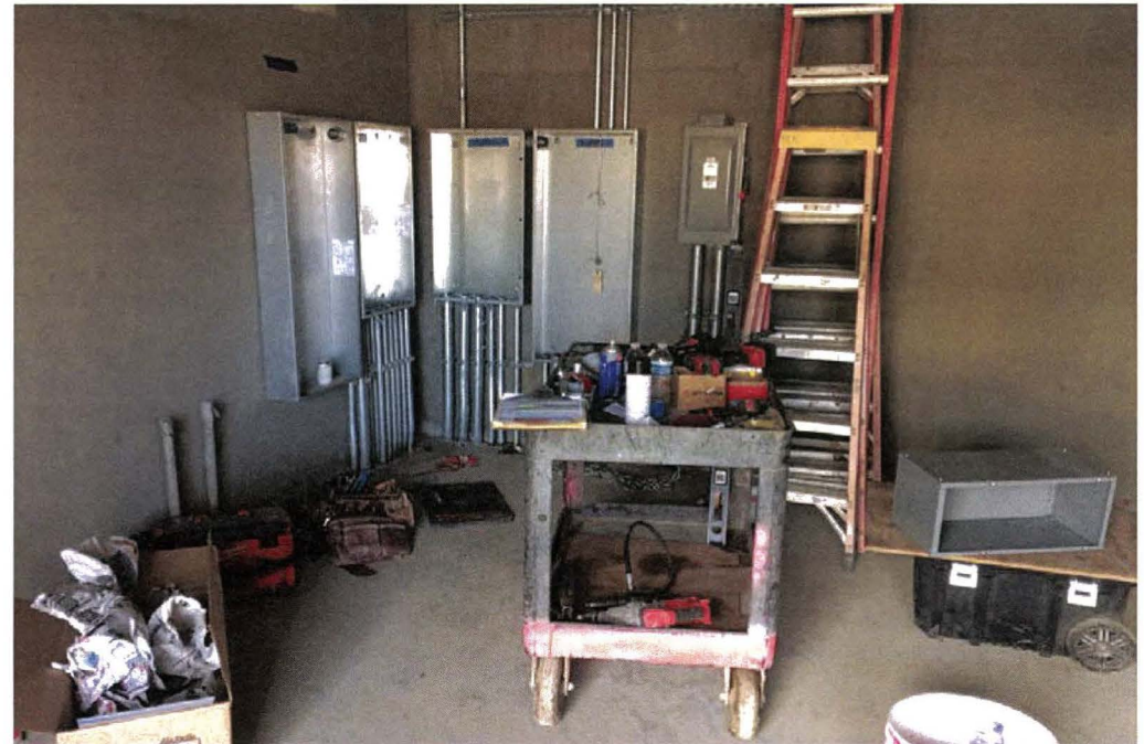
AVIATION/CENTURY BRIDGE – Panels, PPA, PPC, LCPA and LPA installed in the service building electrical room.
