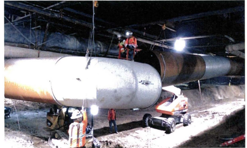
Wilshire/La Cienega Station Temp Ventilation System
