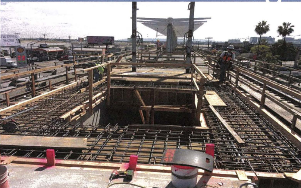
AVIATION/CENTURY STATION – Station platform overhang formwork installation at the service building exit corridor staircase.
