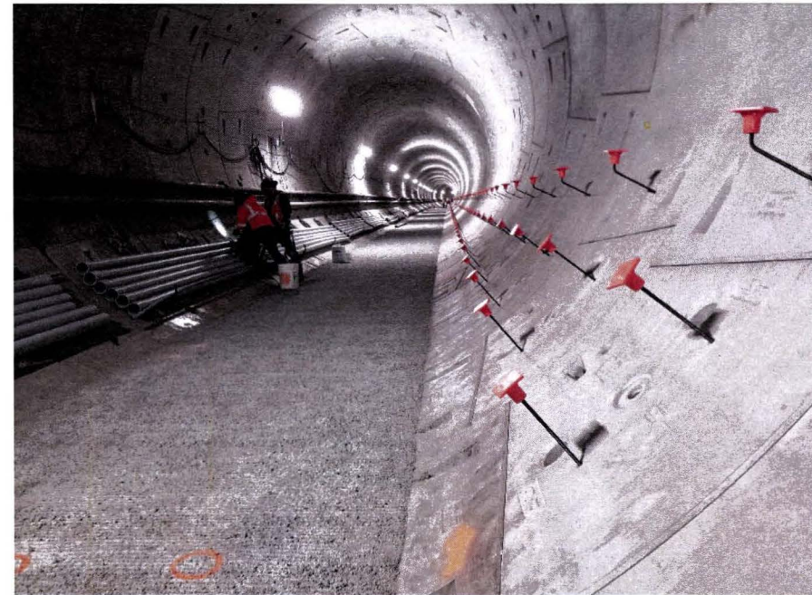
Invert pour along tunnel guideway between Grand Av Arts/Bunker Hill Station and 4th/Flower
