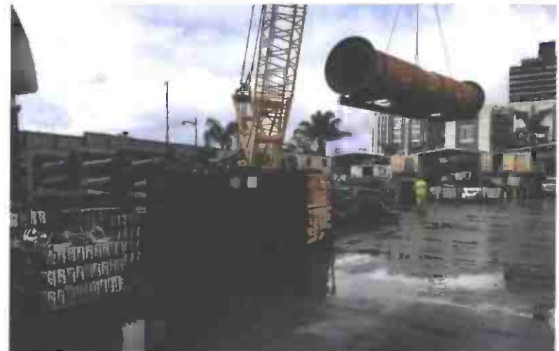
Tunnel Ventilation Booster Fan at North Yard
