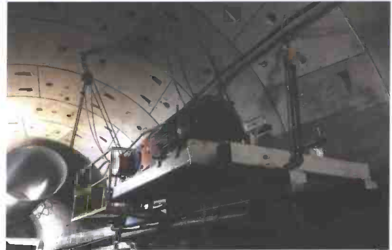
Reach 1 Tunneling – Belt Booster Drive
