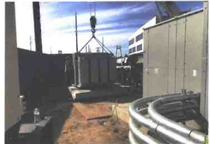
Location 64 Santa Fe Yard – LADWP Transformer
