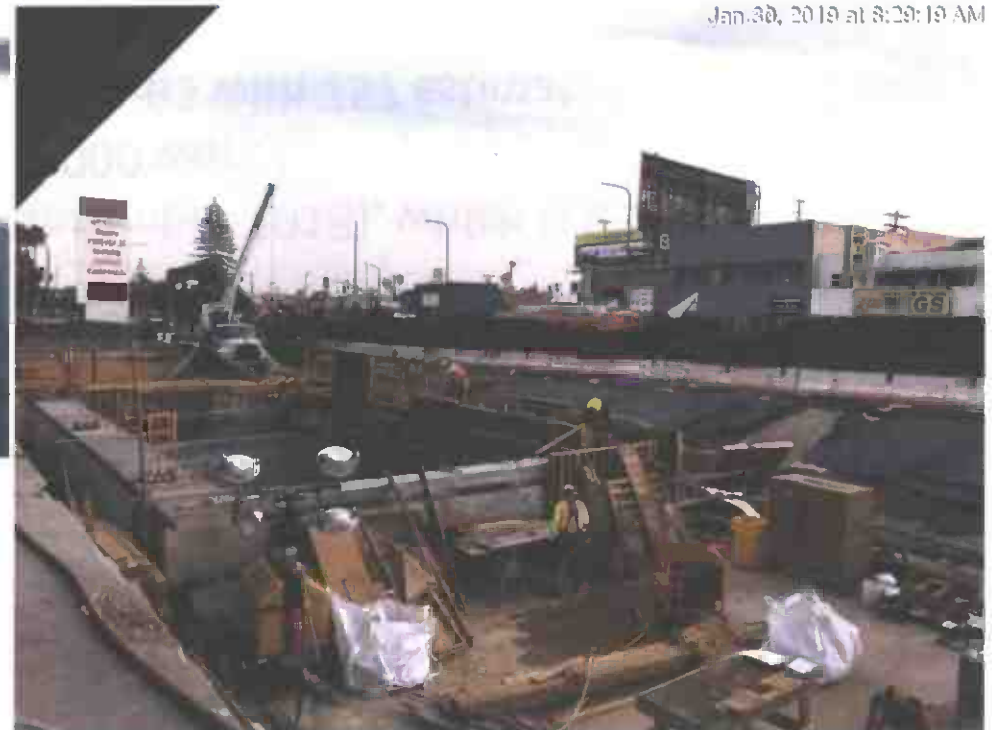
MARTIN LUTHER KING JR. STATION – Installed formwork for walls at the Plaza level
