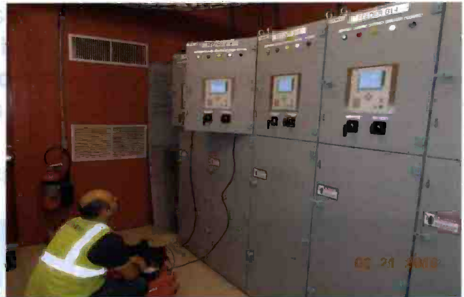
Traction Power Substation (TPSS) #1 – Performing transfer trip test
