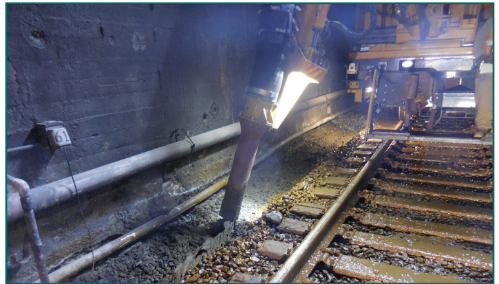
Crews work inside a tunnel along Metrolink's Antelope Valley Line using a RAILVAC excavation machine.
