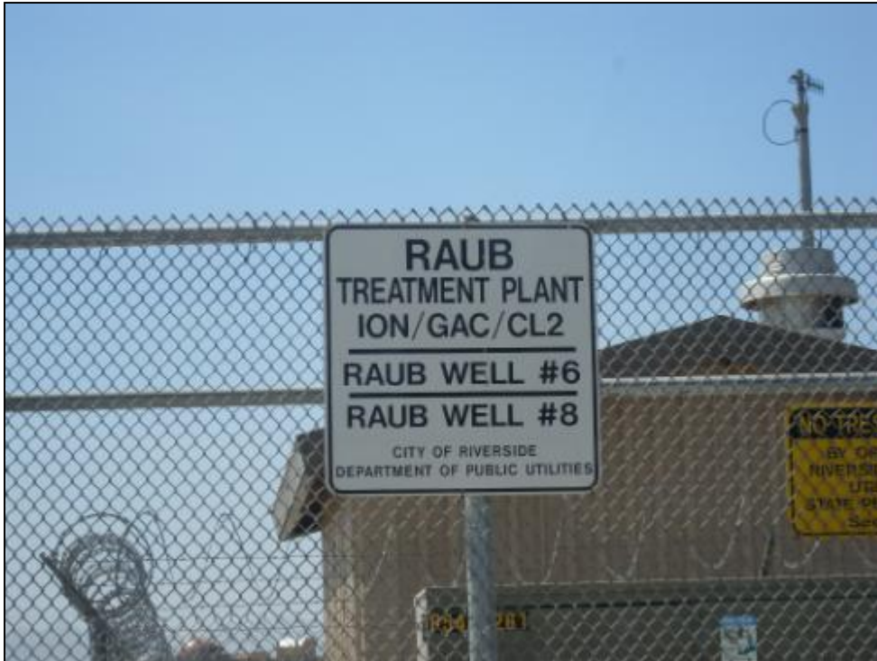
Photo 5: Raub GAC treatment facility located at Waterman Avenue (Map Code AD). View is toward the northwest.
