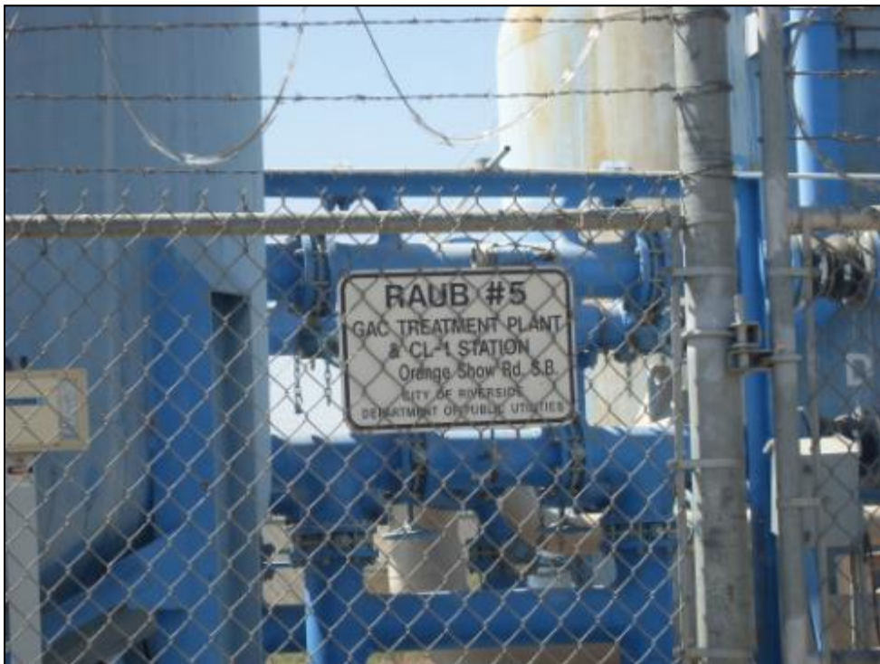
Photo 4: Raub GAC treatment facility located at Waterman Avenue (Map Code AD). View is toward the northwest.
