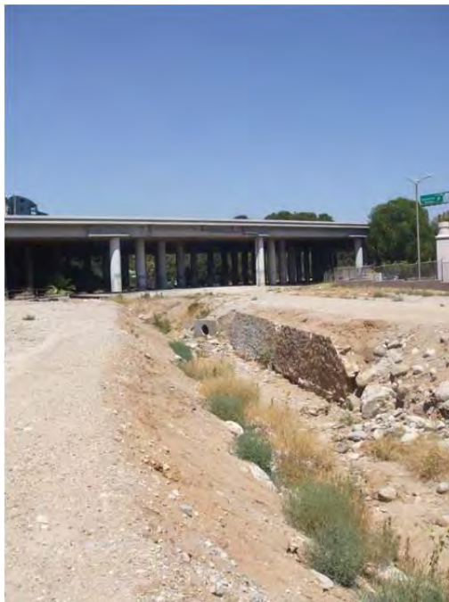
Photograph 6: Concrete drainage feature and fieldstone and mortar wall south of railroad bridge, view to southwest
