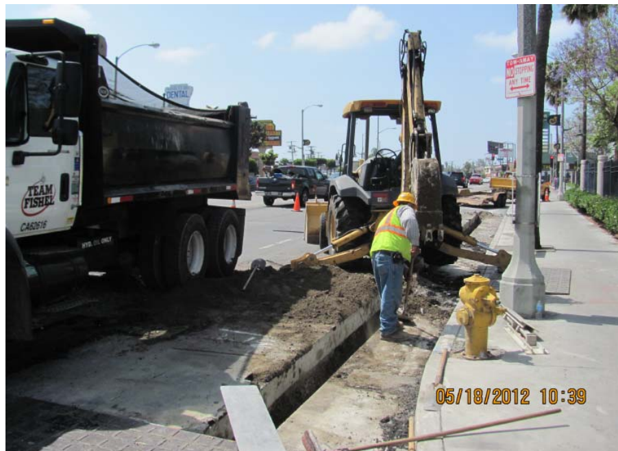
Team Fishel, third party contractor, is beginning utility relocation at Martin Luther King Blvd.
