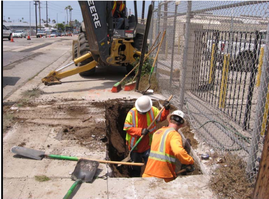
VCI, third party contractor, is excavating for vault installation at Arbor Vitae.
