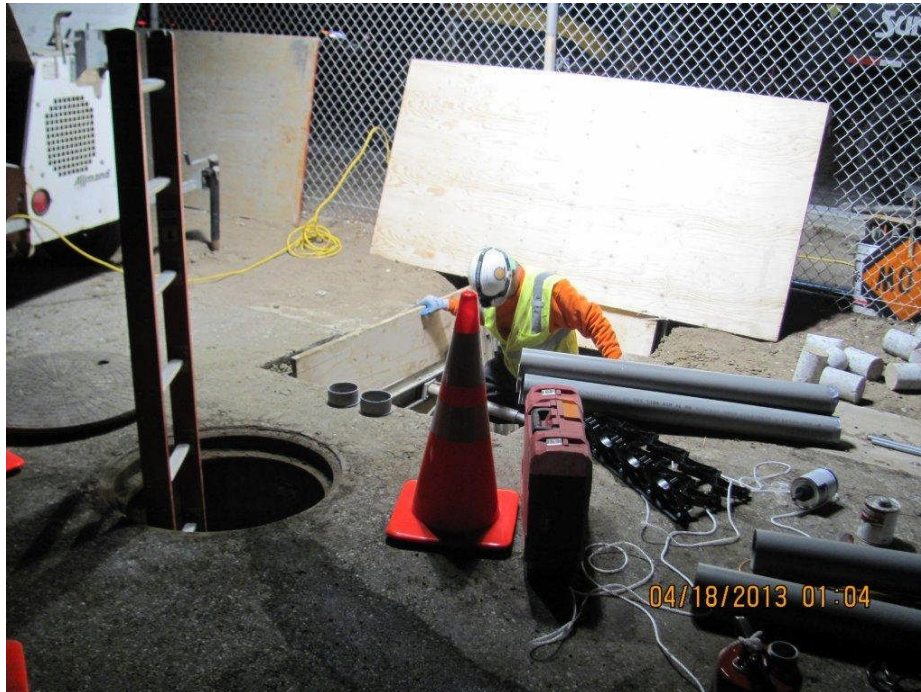
Advanced utility Relocations contractor installing conduit stub out at FAA manhole east of Aviation at 25L
