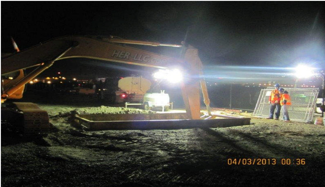
Advanced Utility Relocations contractor backfill and compaction of jack and bore pits 25L.
