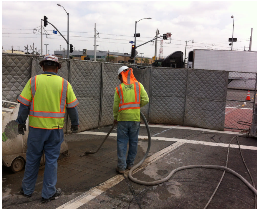
Potholing by AT&T (Irish) using Sound Blanket at 1 st Street and Alameda
