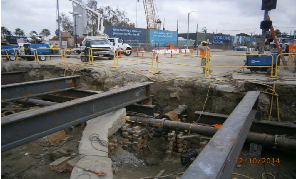
Steel Sleeve on Gas Main.
