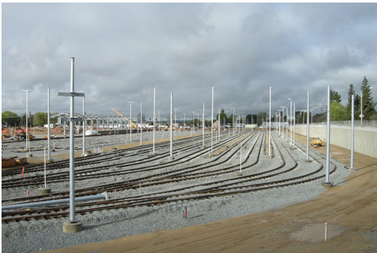
Operations Campus: OCS and Site Lighting Poles erected throughout the North Storage Track areas
