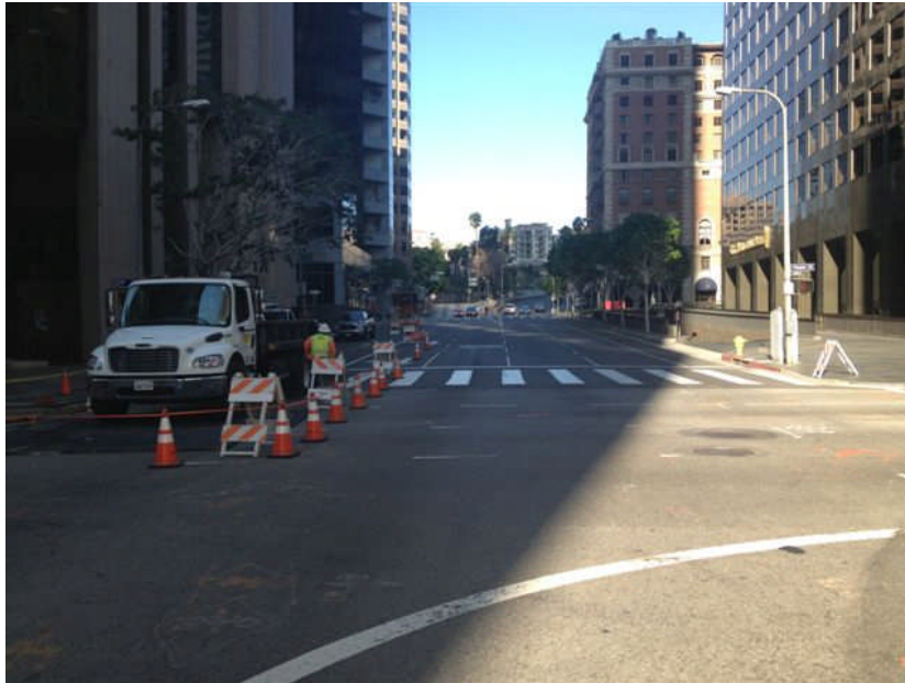
Sixth Street and Flower – Traffic control in place by Irish Construction for Level 3 Relocation
