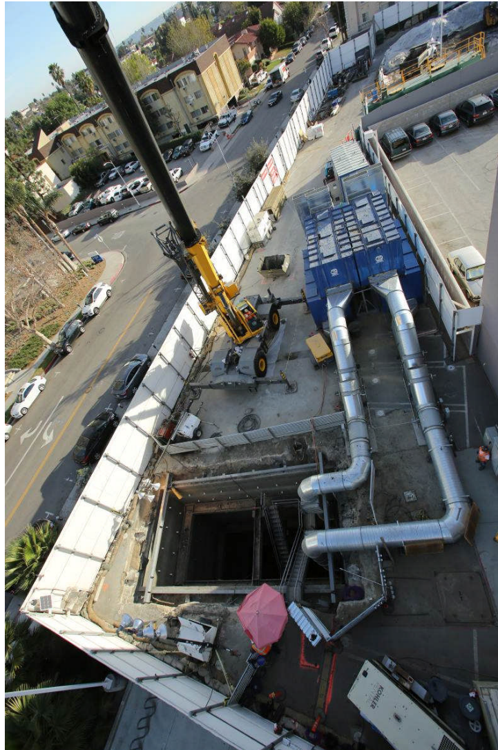
View of Exploratory Shaft Ventilation Ducts and Carbon Scrubbers
