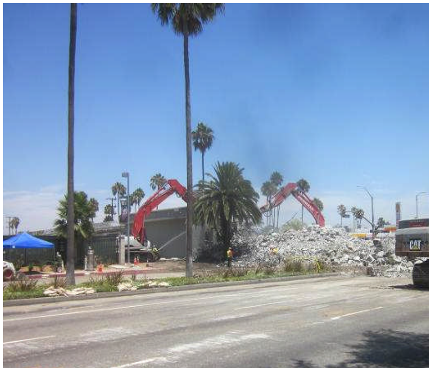
Century bridge rubble pile from the bridge deck on July 26 th .
