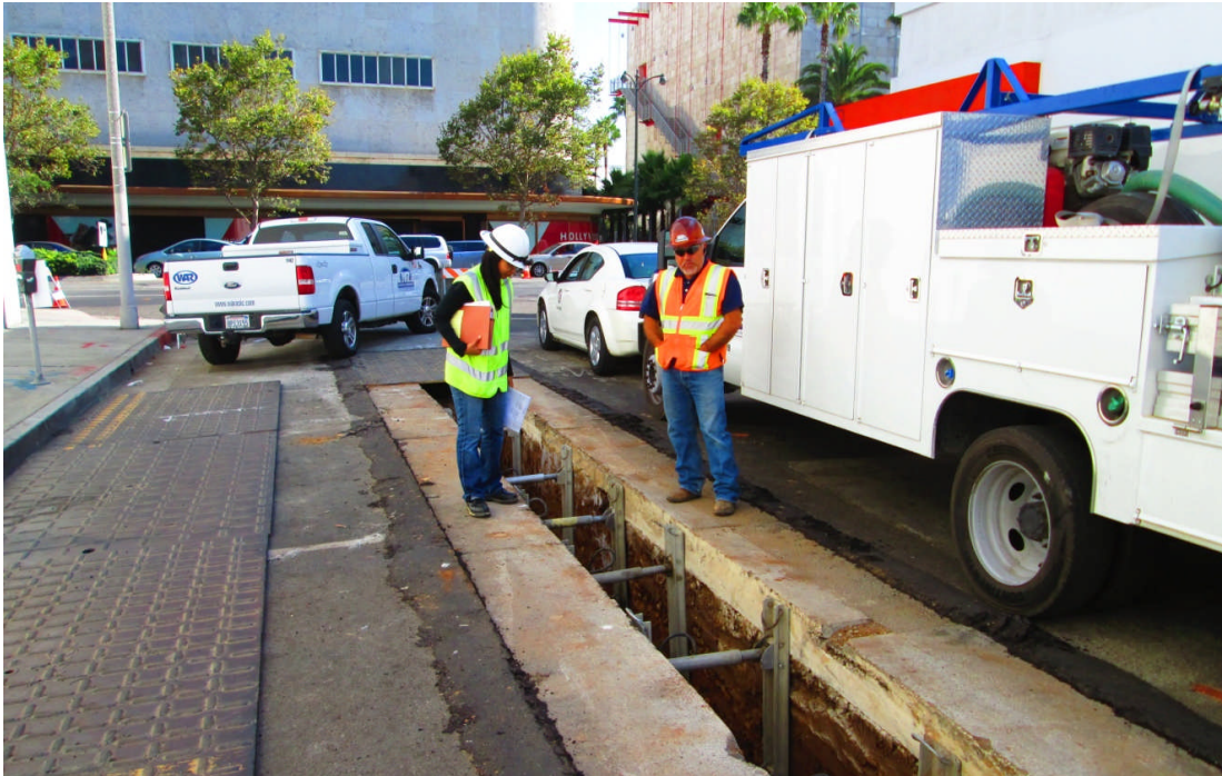
LADWP Inspecting Work of C1055 Contractor on Orange Grove Avenue in the City of Los Angeles
