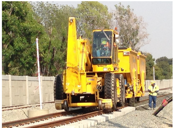
Segment 3: East of Buena Vista - Flooding Ballast
