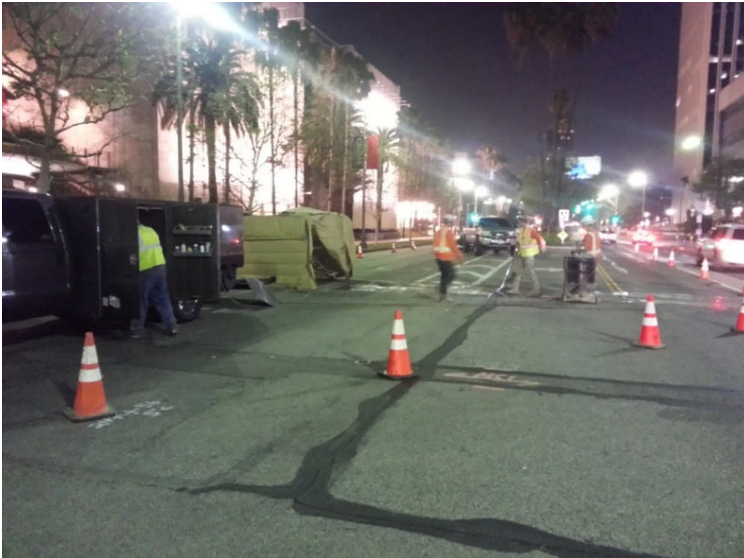
Saw-cutting Pavement using a Noise Blanket Cart near the Wilshire/Fairfax Intersection in Advance of Relocating Utilities
