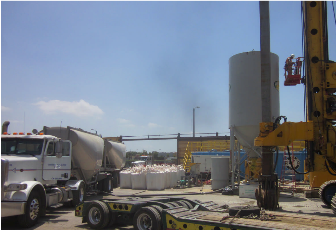
Filling cement silos for Cutter Soil Mixing (CSM) operation in the Crenshaw/Exposition Station yard.
