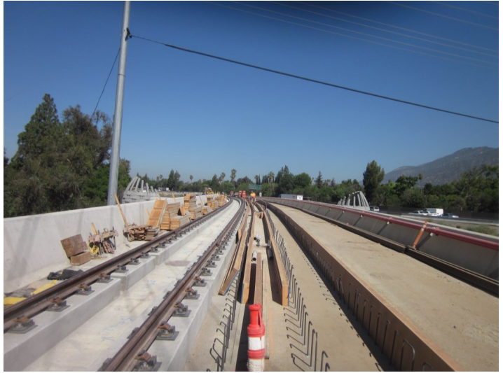
Segment 1: IFS Emergency Walkway and Ductbank
