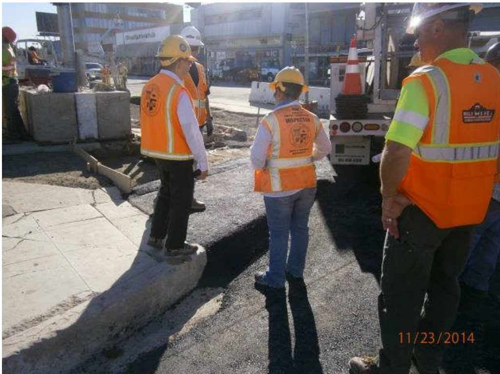
City of Los Angeles – BOE on site inspecting work south of Rodeo.
