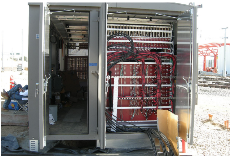
Operations Campus: Train Control Bulgallow Wiring
