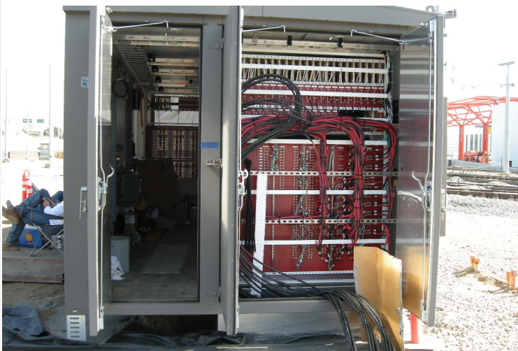
Operations Campus: Train Control Bulgallow Wiring
