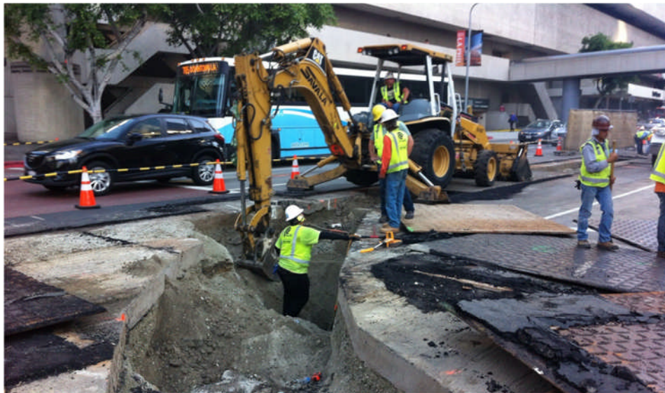
DWP Power trench excavation at the intersection of Flower Street and 5 th
