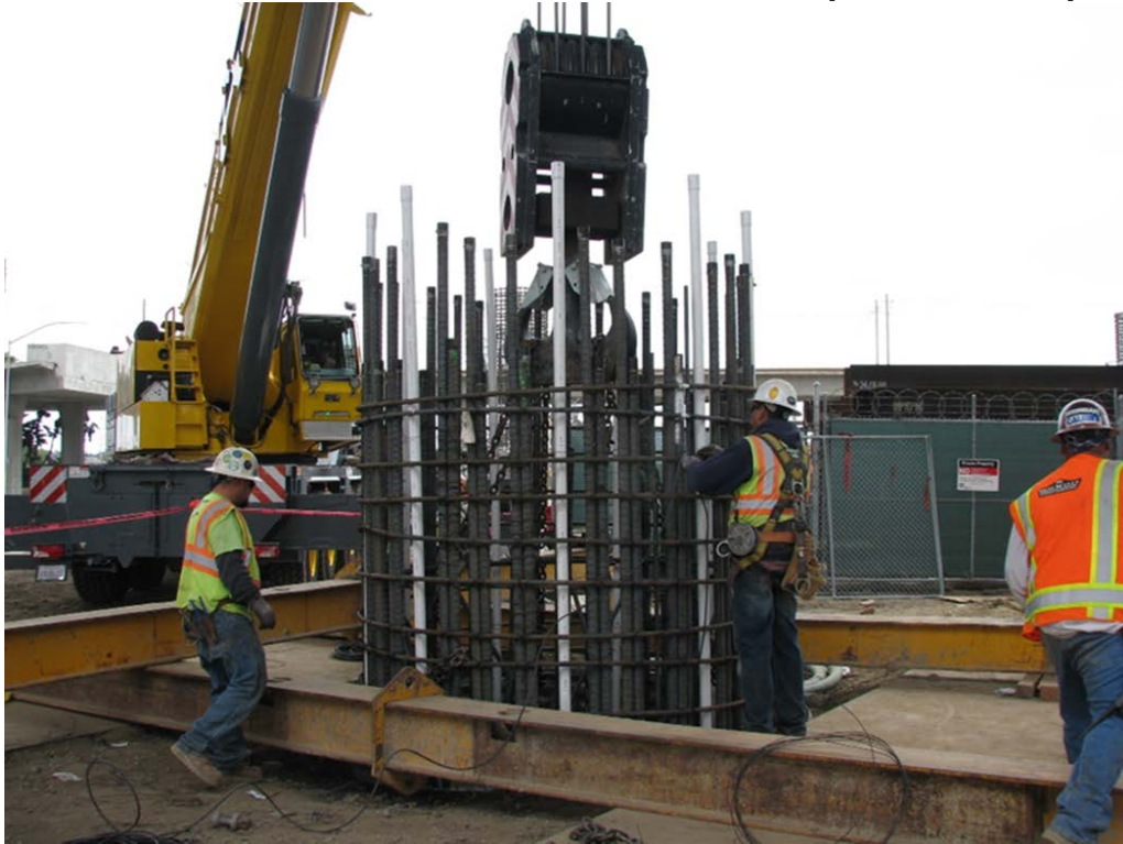
Green Line Tie-In Bridge-Installation of Rebar Cage for Bent 3E CIDH (3 rd Section with 4 th Splice).
