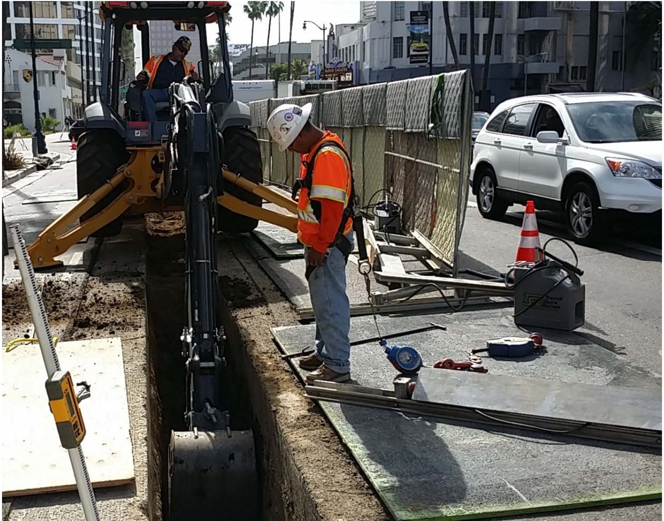
C1056 Wilshire/La Cienega AUR Contractor Excavating SCE Power Ductbank East of La Cienega Boulevard
