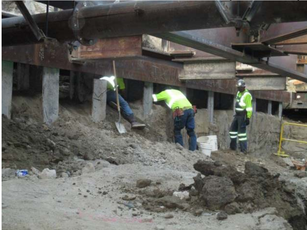
Removing Soil and Placing Lagging on the north wall of the Expo Station.
