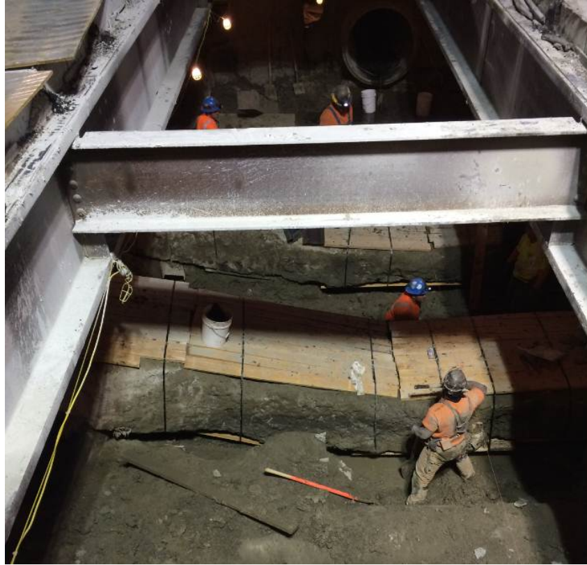
Expo Station Utility Support.
