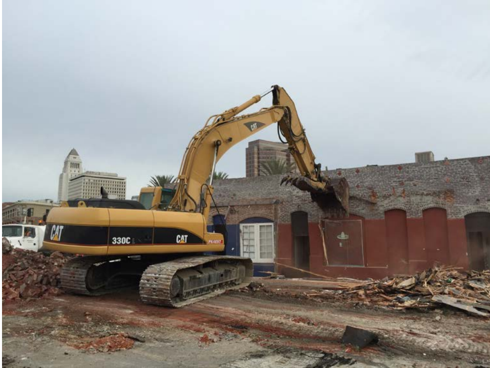
C0980 Contract – Demolition of Senior Fish Building at 1 st and Alameda Sts.
