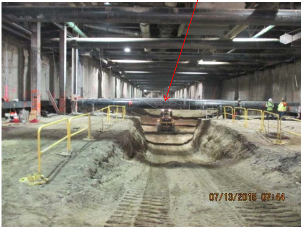
EXPOSITION STATION – Excavation of trough within the Expo station box looking south.
