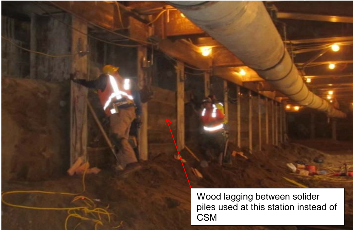
VERNON – Installation of lagging along the west wall within the station box.
