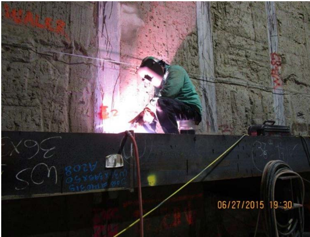
EXPOSITION STATION – Welding Tier 2 Bracing along the West Wall in the south Station.
