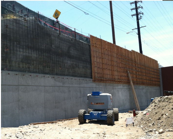
Construction of fractured fin form for CIP Wall on Irwindale Parking Structure Soil Nail Wall
