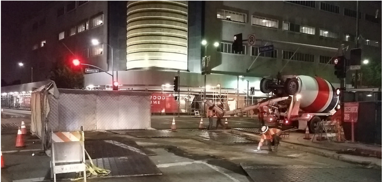
C1055 Wilshire/Fairfax AUR Contractor Restoring Pavement for Power Trenches at Wilshire/Fairfax Intersection
