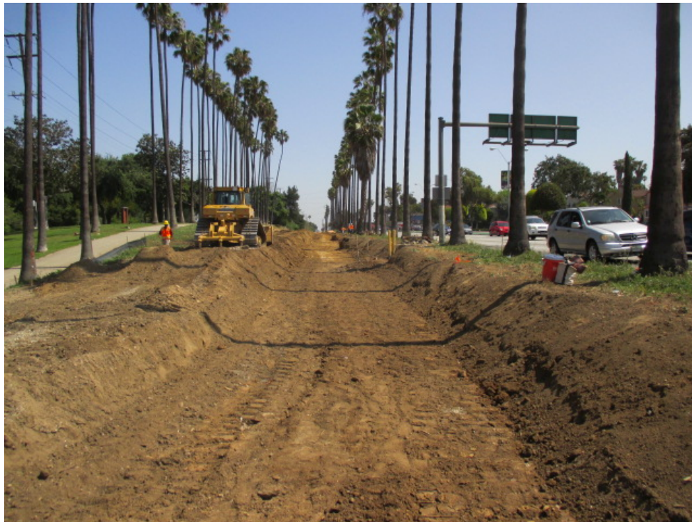
Florence Between Centinela and Redondo Clearing for Guideway Installation and Utility Investigation.
