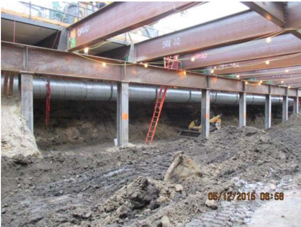
Undermining CMP Storm Drain at MLK.
