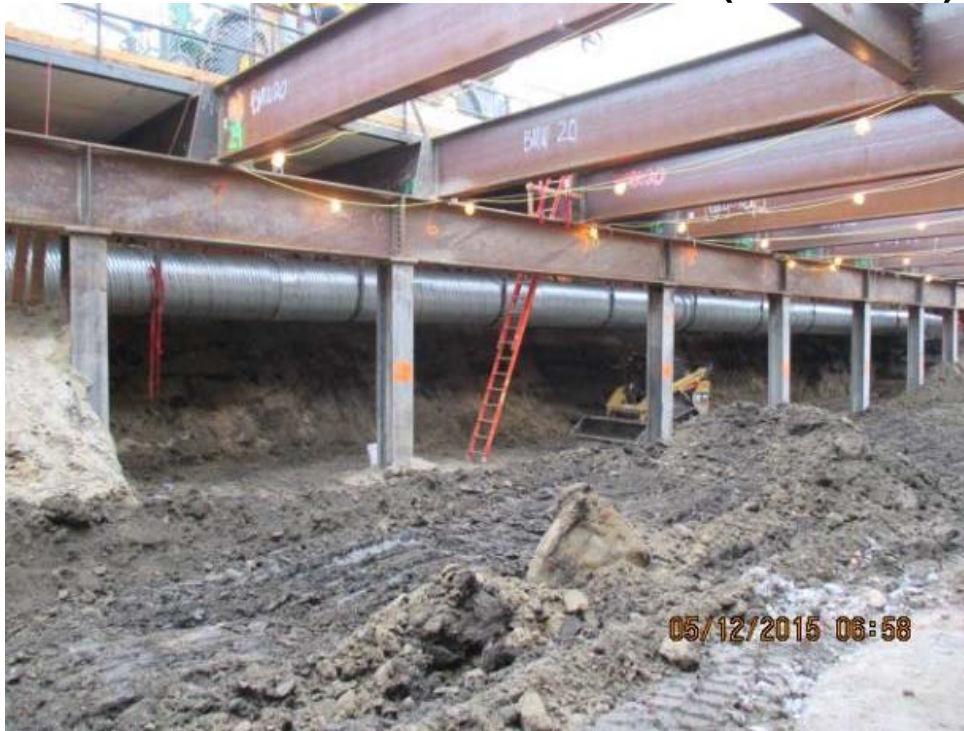
Undermining CMP Storm Drain at MLK.
