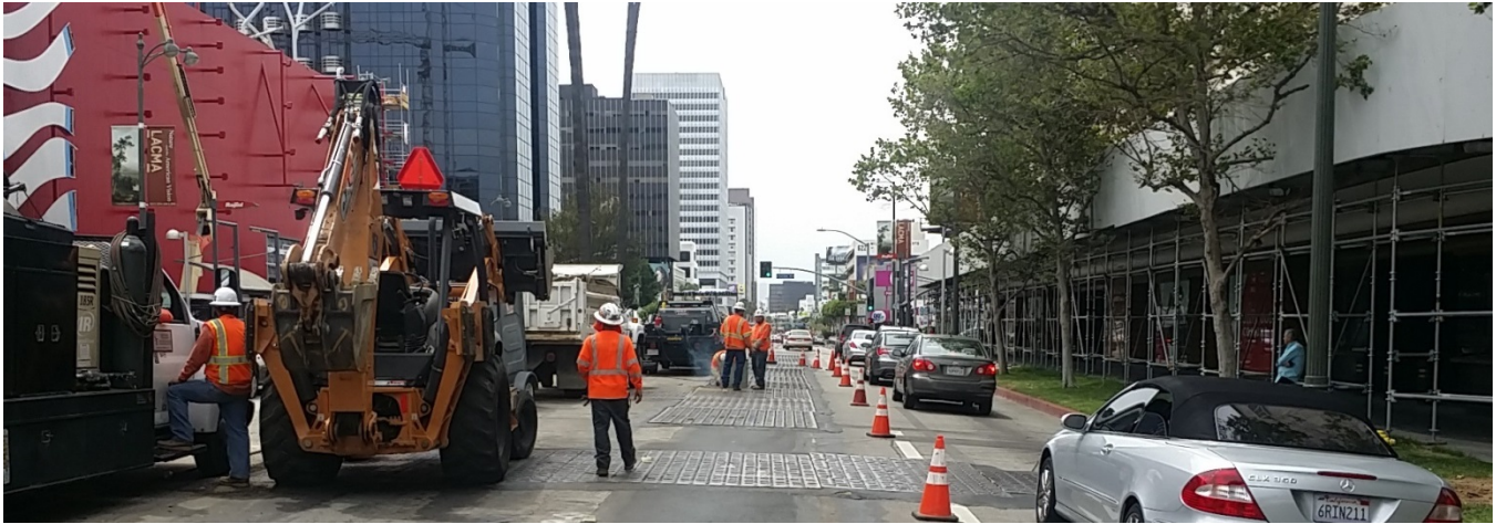
C1055 Wilshire/Fairfax AUR Contractor Placing Steel Plates with Traffic Control in place along Wilshire Boulevard
