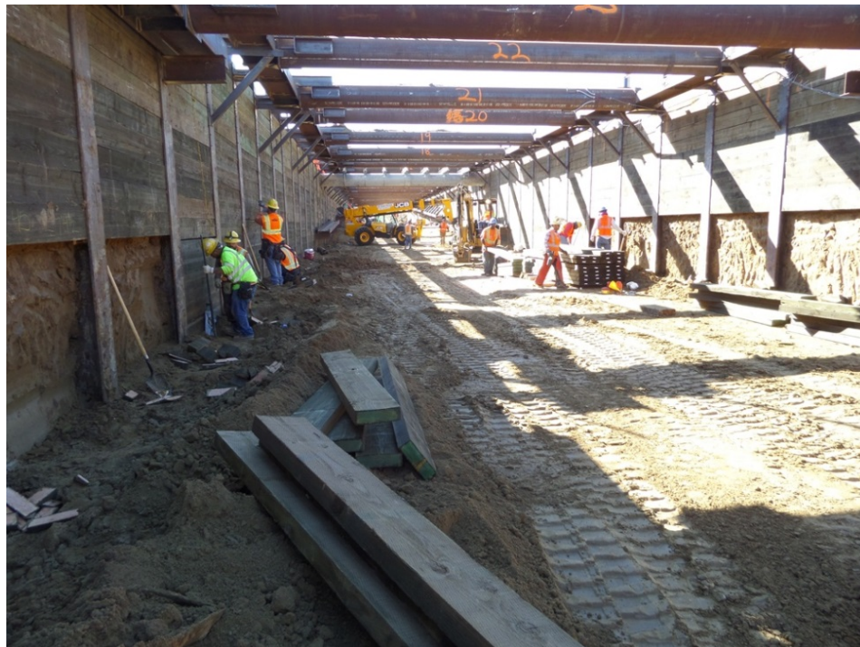
UG#1 - Struts and wales being installed per plan. Tier 2 lifts and kickers being installed in preparation for tier 2 walers and struts. Treated lagging installation ongoing as excavation continues.
