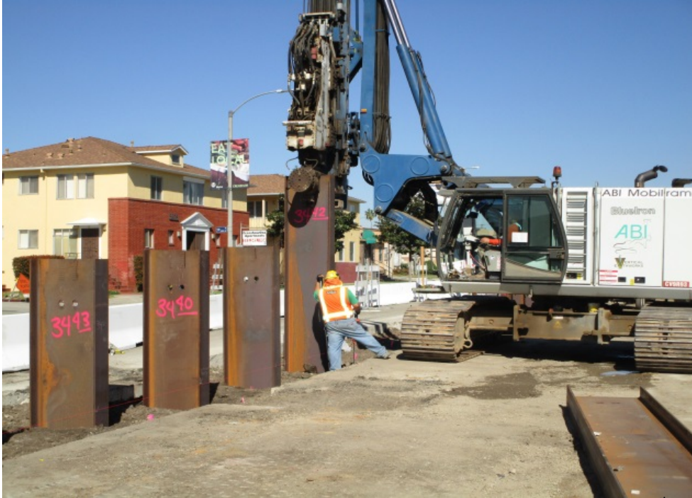
UG3 – Vibrating piles at UG3 looking north (Near Crenshaw and 58 th Pl.).
