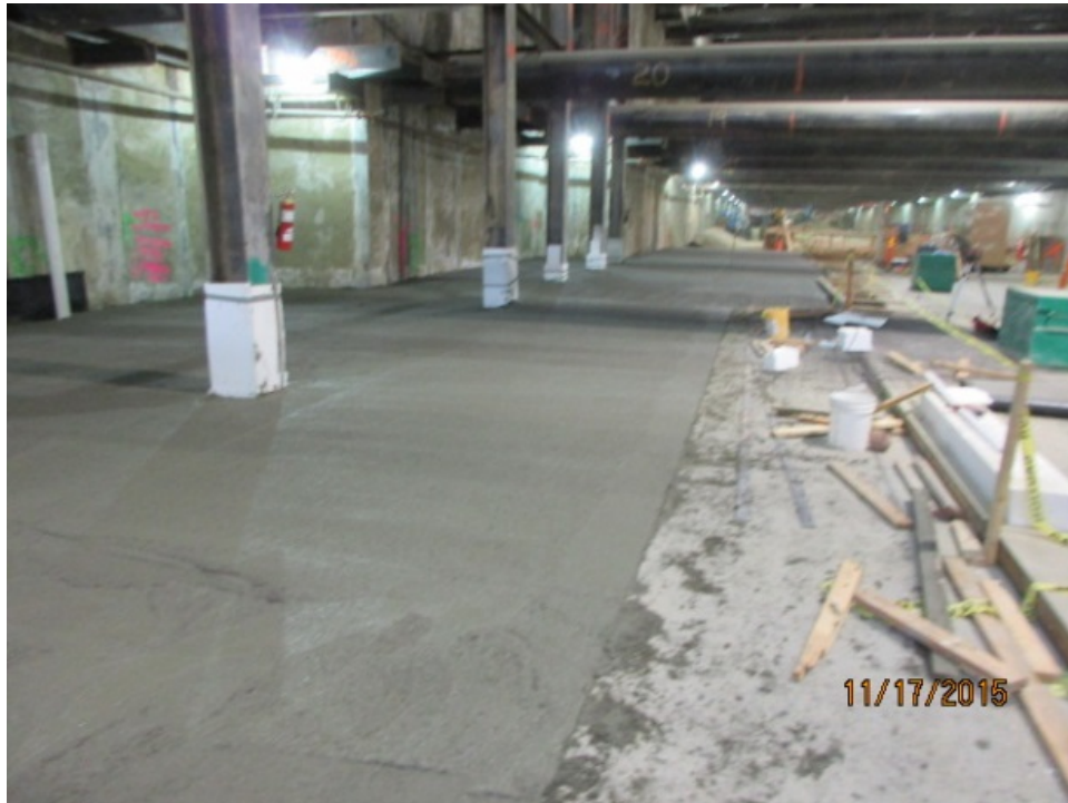
EXPO/CRENSHAW STATION – Phase 2 mud slab installed at the central portion of Expo station box.
