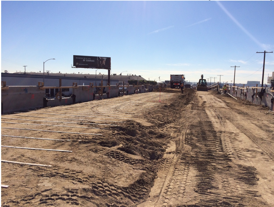
MSE (Wall 3, 60L&R): Precast Panel erection, placement of soil reinforcement, backfilling and compaction testing ongoing.
