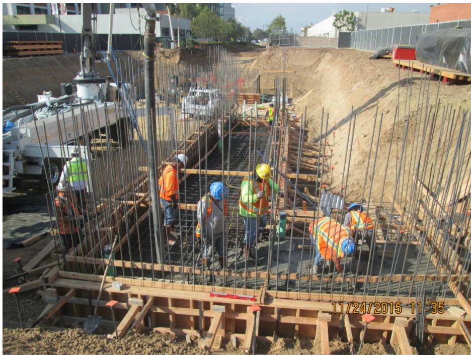
FAITHFUL CENTRAL BIBLE CHURCH - Pedestrian Underpass: Wall steel placed for tunnel/walkway structure.
