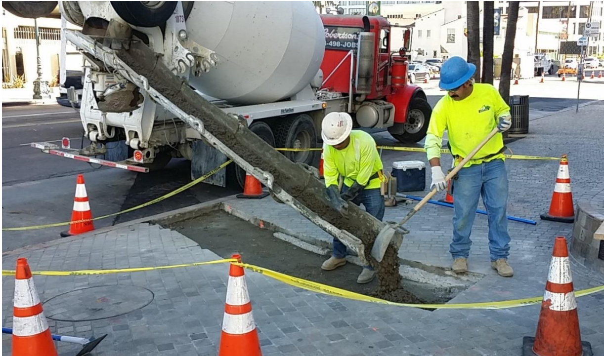
C1056 Contractor Restoring Sidewalk over Southern California Edison's Ductbank East of La Cienega Boulevard
