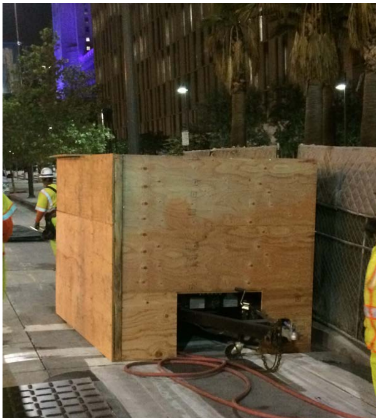
Enclosing air compressor at 2 nd /Spring to lower noise level
