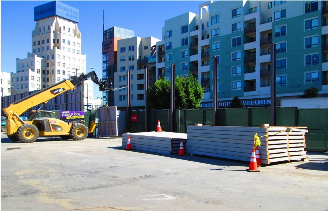
C1045 Contractor Installing Soundwall Panels at the South Wilshire/La Brea Construction Staging Site
