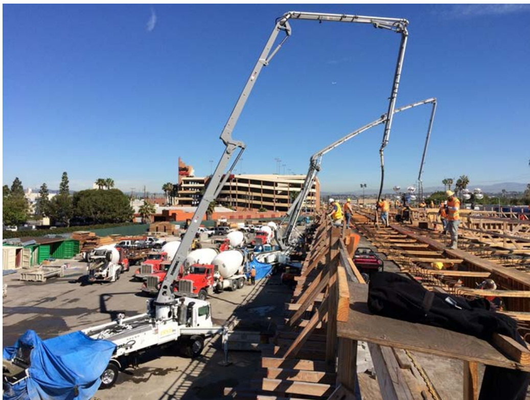
AVIATION/CENTURY BRIDGE – Placed concrete for the girder stems and soffit at Frame 1A.
