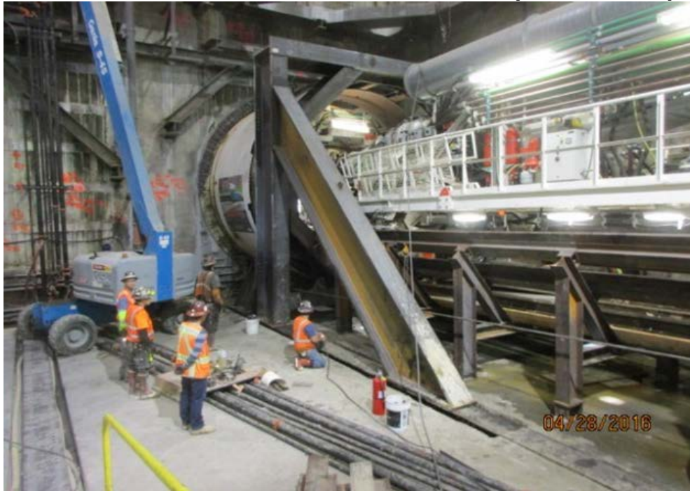
EXPOSITION/CRENSHAW STATION – Advancing TBM and thrust frame. The TBM is buried up to the tail-can.
