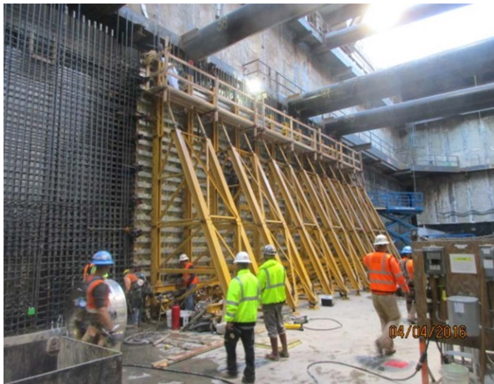
EXPOSITION/CRENSHAW STATION - Placement of 1 st section of lower station wall (east side of station box).
