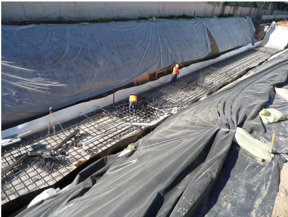
FAIRVIEW HEIGHTS STATION – Crews installed the HDPE membrane; MEP embeds and invert rebar.
