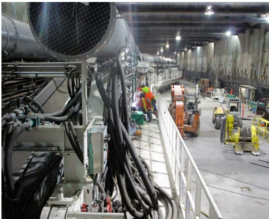
EXPOSITION/CRENSHAW STATION – Looking north from the TBM towards the trailing gear gantries.
