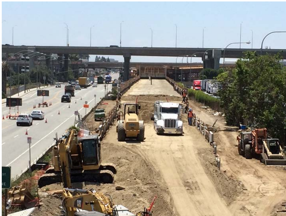
MSE WALL 17L & R (North of Imperial Highway) – Subgrade preparation, leveling pad placement, precast panel erection, embankment backfill and compaction.
