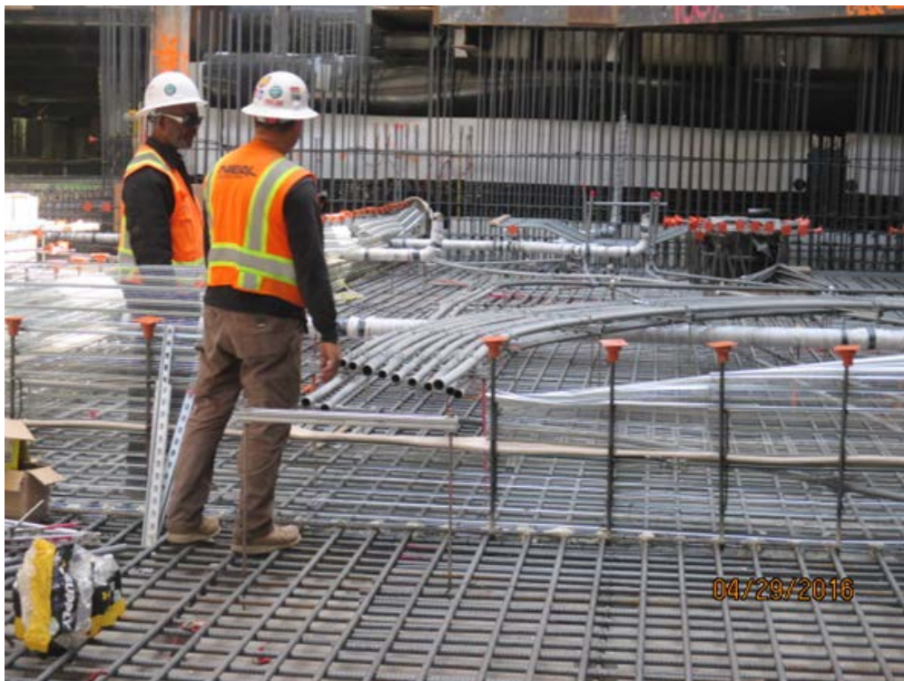
MARTIN LUTHER KING JR. STATION - Installation of electrical conduits, plumbing and rebar.
