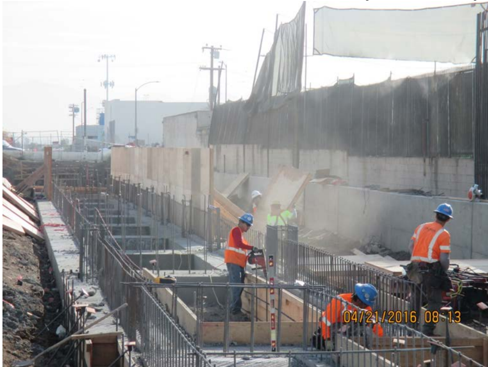
FAIRVIEW HEIGHTS STATION – Station foundation footing completed. Crews worked on installing stem wall forms and rebar.
