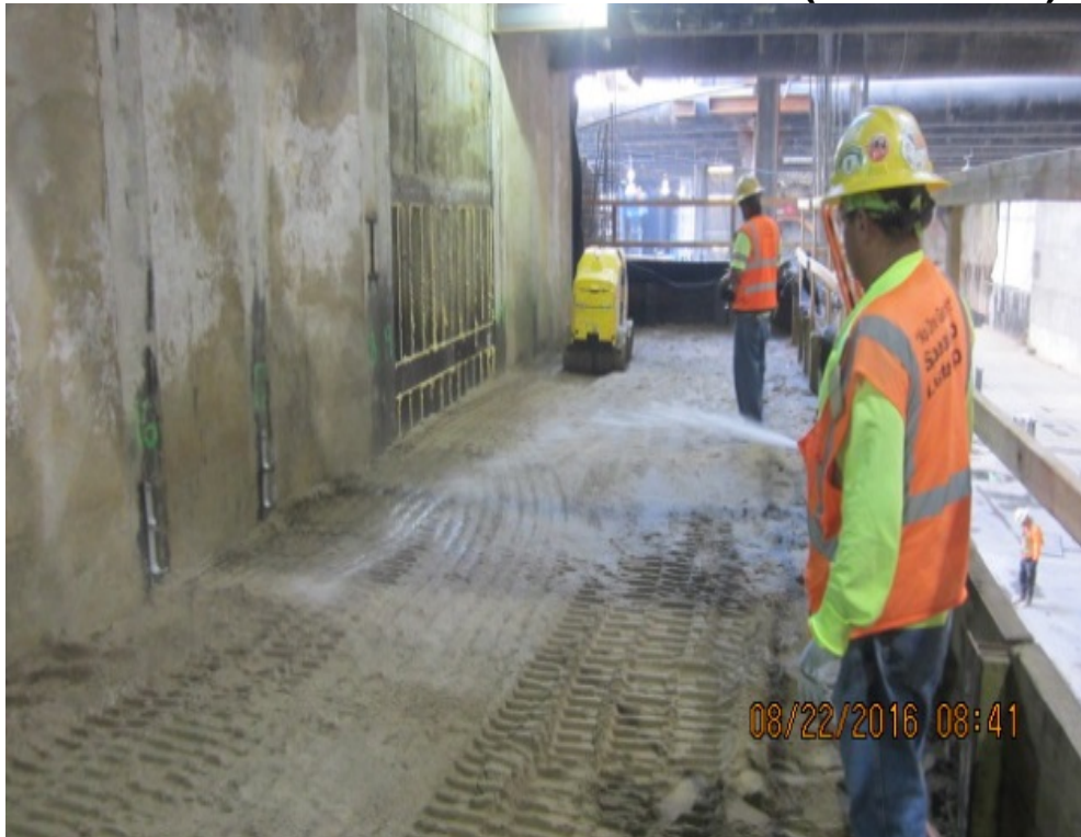
MARTIN LUTHER KING JR. STATION – Backfill and compaction activities at the south west bump out wall.
