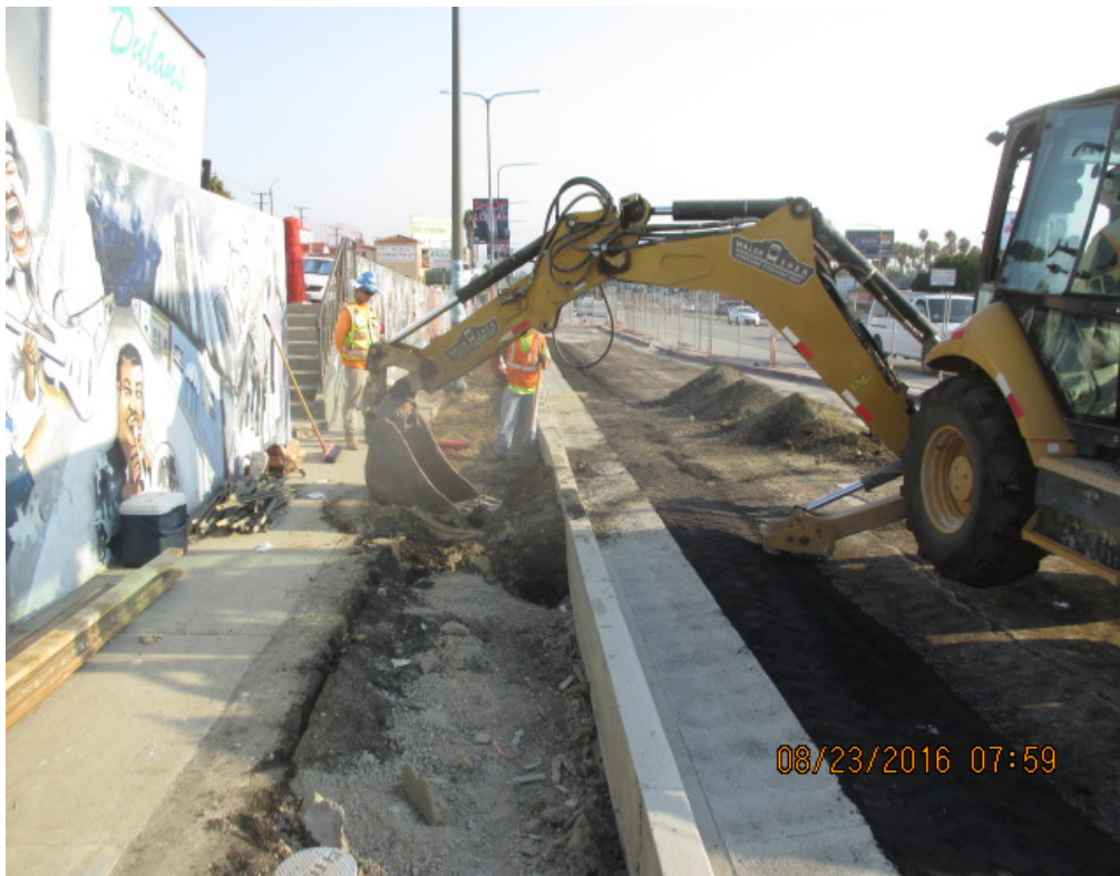
PARK MESA – Back fill activities behind installed curb and gutter at mural walls.
